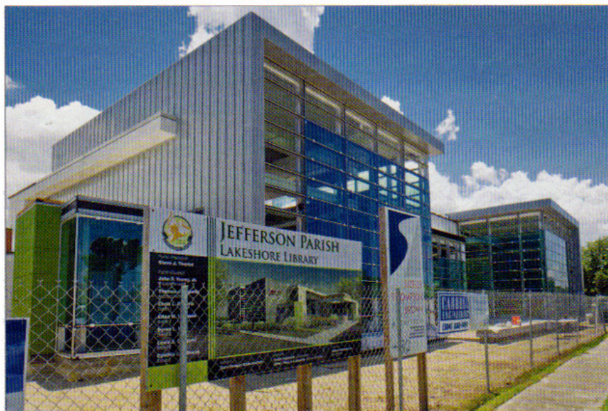
Construction is underway on replacements for several of the libraries destroyed by Hurricane Katrina, including Jefferson Parish Library's Lakeshore branch.
